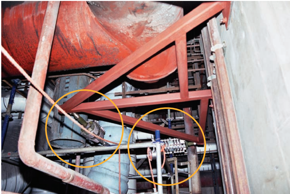
FIGURE 1 – Turbine Pedestal WEAR™ Supporting Structure
